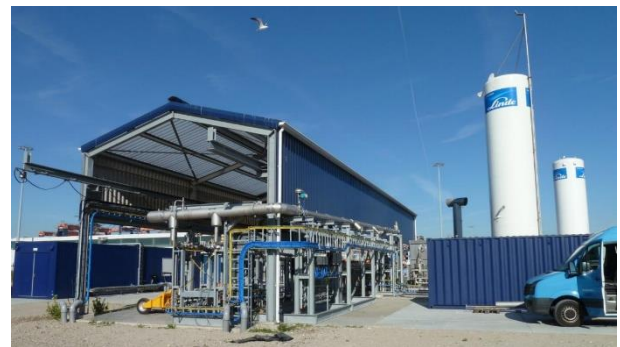
Figure 11: LNG calibration and test facility (VSL) [11]
