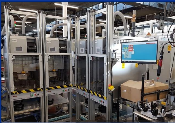
Equipment for Meter Manufacturer Test facility for domestic gas meters. Complete smart meter calibration.
